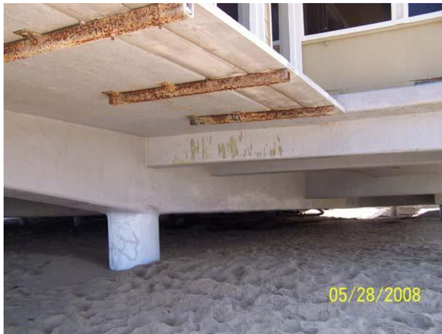
Figure 7: Some paint peeling from FRP on the beam.
