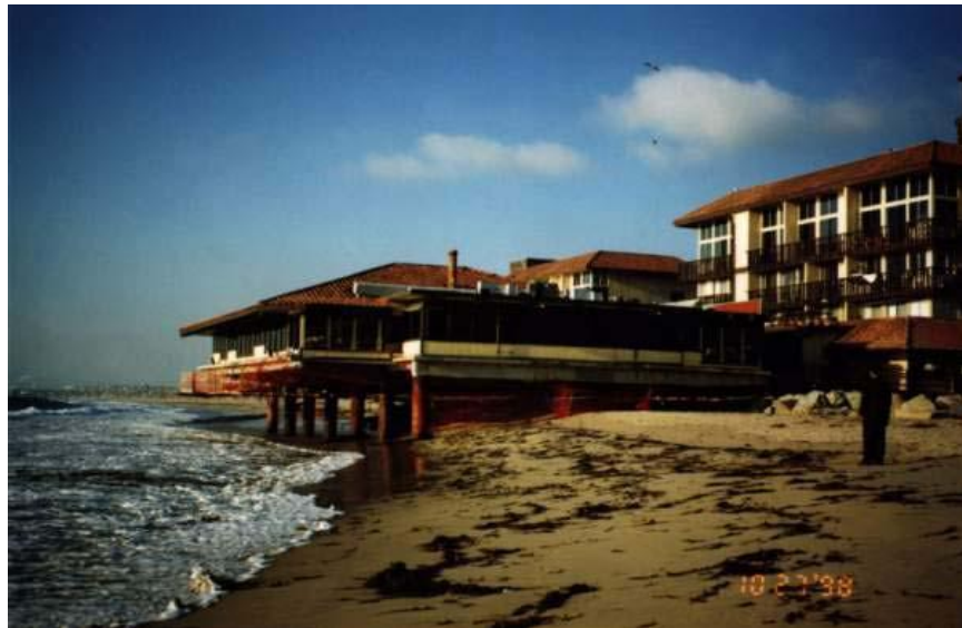
Figure 1: Un-repaired restaurant with poor conditions.
