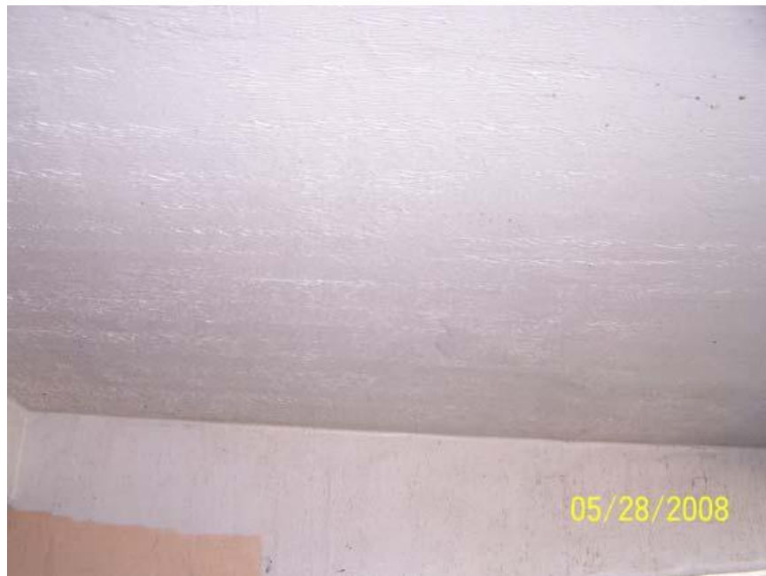
Figure 9: Repaired slab without defects after 9-year of services
