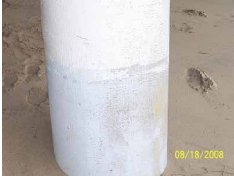
Figure 6: a column with some coating worn out on the side facing the sea due to the abrasive action of sea water with sand. The small yellow area shows the FRPs under the coating
