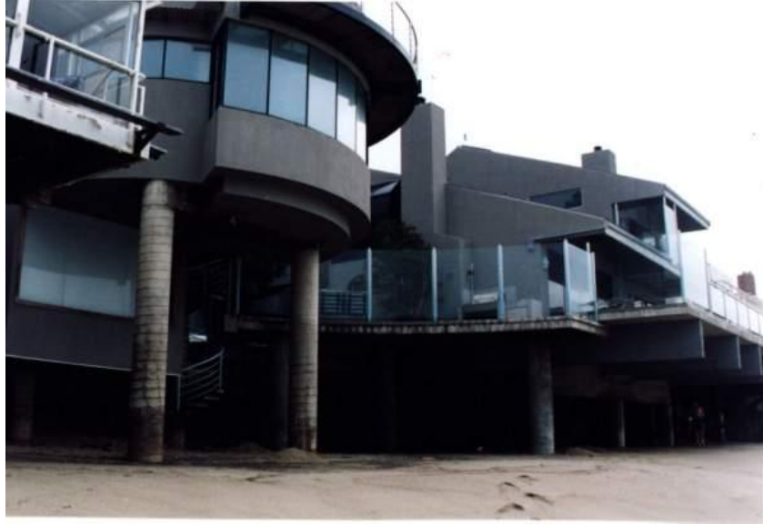
Figure 3: The ASR deteriorated concrete columns, with extensive cracks on the concrete surface and concrete chalking (on the bottom of the column).
