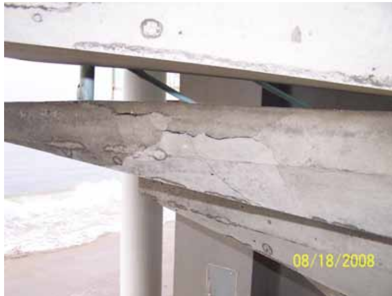
Figure 9: Concrete steps in the same building. Note the back column was retrofitted with Tyfo ® Fibrwrap ® systems.
